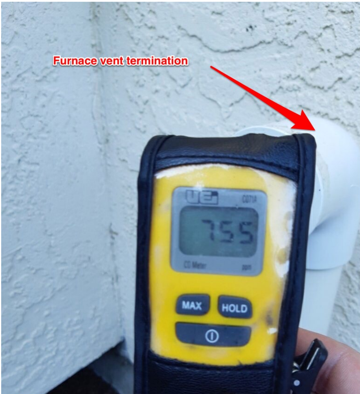
Image 11 – Carbon monoxide meter registering 755 parts per million (ppm) at the furnace vent termination while the furnace was operating.
