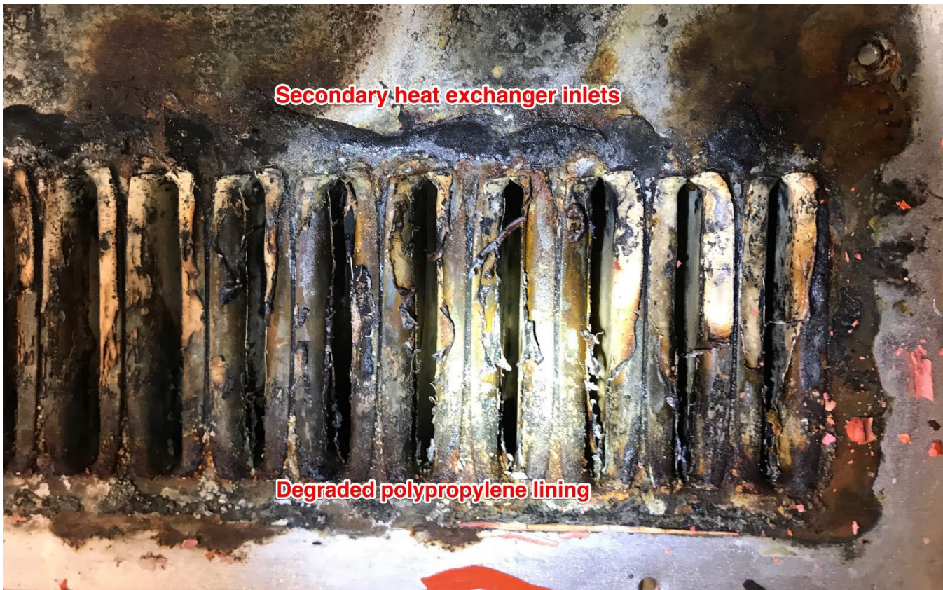
Image 9 – Replacement secondary heat exchanger tubes inlets after under 5 years of operation.
